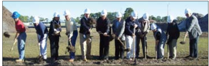
Sun 'n Lake Board of Supervisors, General Manager and representatives from Lodge Construction, Weller Pools and The Evans Group break ground on the new recreation complex
